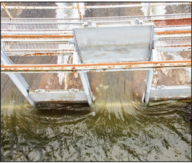
In order to complete dam maintenance, TVA workers are opening several spillway gates at a time to release water from the lake into the Nottely River. Photo by Shawn Jarrard
